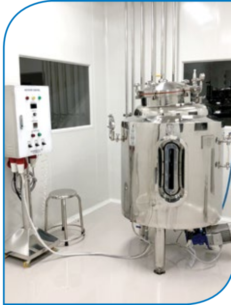
DISPENSION TANK OF INJECTION SOLUTION
